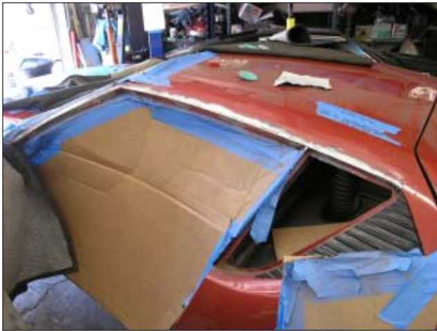
Above: The rain gutters have been removed and smoothed out. Below: Steel panels were shaped and welded-in the cowl.
