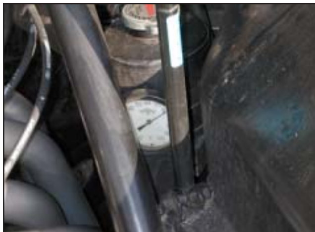
Above: Reservoir mounted temperature gauge permits remote viewing of system temperature.
